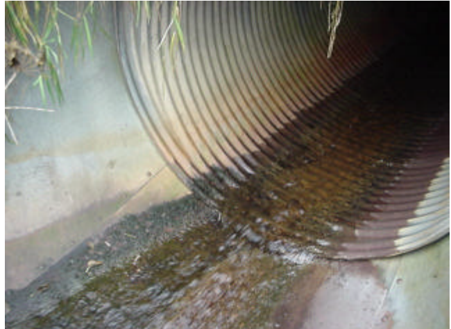
Figure 15 - Bay Creek culvert with algae growth on bottom of pipe
