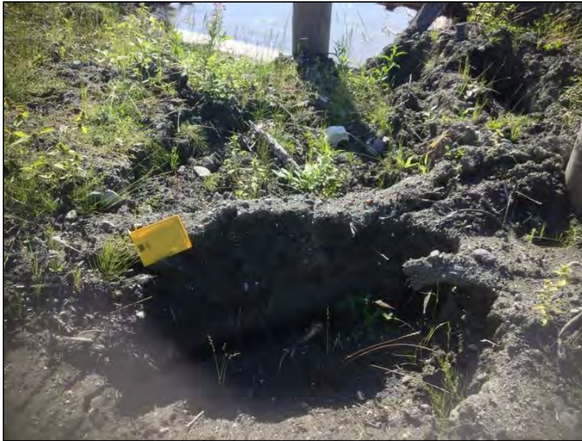
Figure 7. Void formation and slumping at upstream end of wood revetment, Klukwan, Alaska, (ADOT&PF, August 2013).
