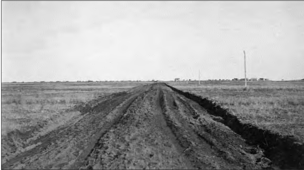
Figure 21. Initial road construction prior to regrading. Photo c.1910. Source: Archives, University of Alaska, Fairbanks.
